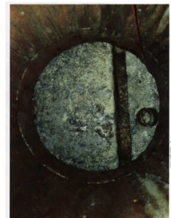
Heavily used grease interceptor
